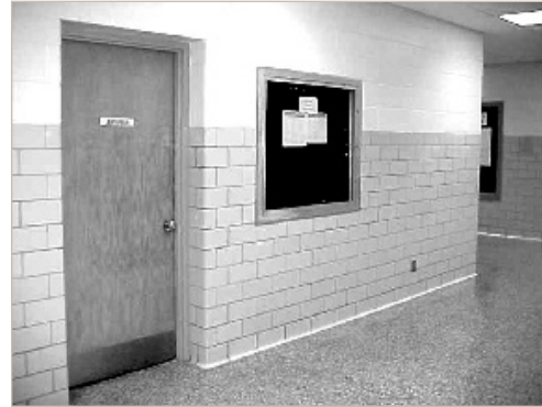
No interlock in a typical school door
